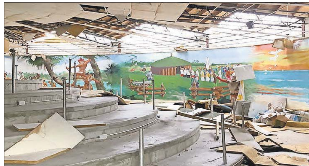
The interior of the badly damaged cyclorama building at Warm Mineral Springs shows murals painted on the walls that some want to salvage.
